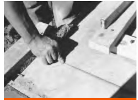
Fig. 7: Trace building wall lines. Check alignment and square. Snap chalk-line on slab along the inside face of the wall panels.
