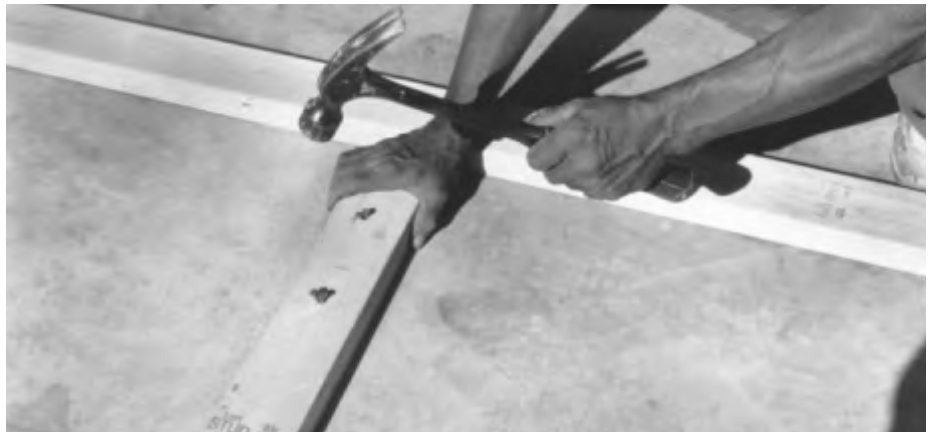
Fig. 8: Place cleats every 4 ft. and perpendicular to wall lines. (secure cleats with masonry screws Hilti, ITW Tapcon or similiar).
